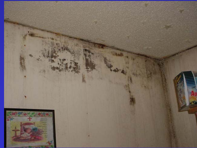
Mold due to leaky roof
