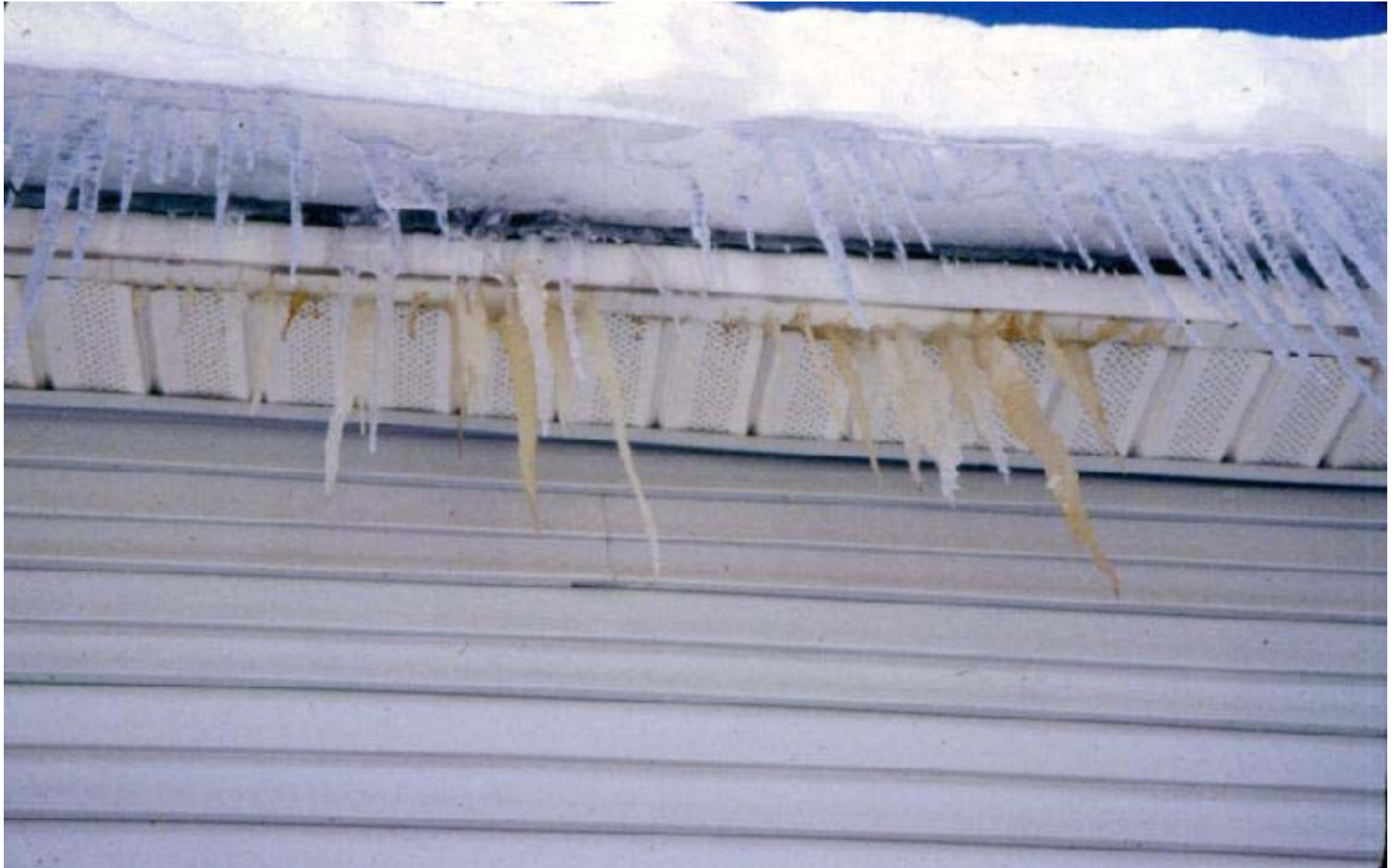
Exercise 5: Identify the Moisture Problems
