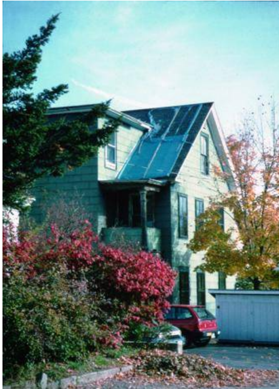
Exercise 5: Identify the Moisture Problems
