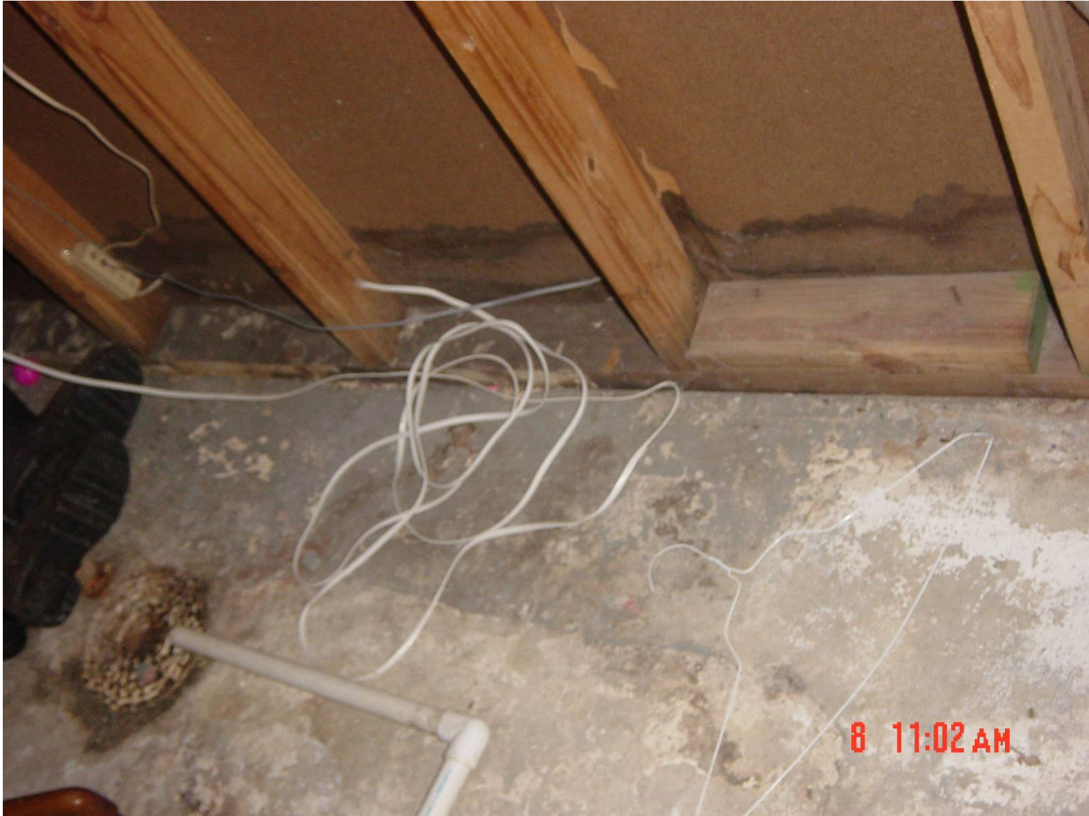
Exercise 5: Identify the Moisture Problems
