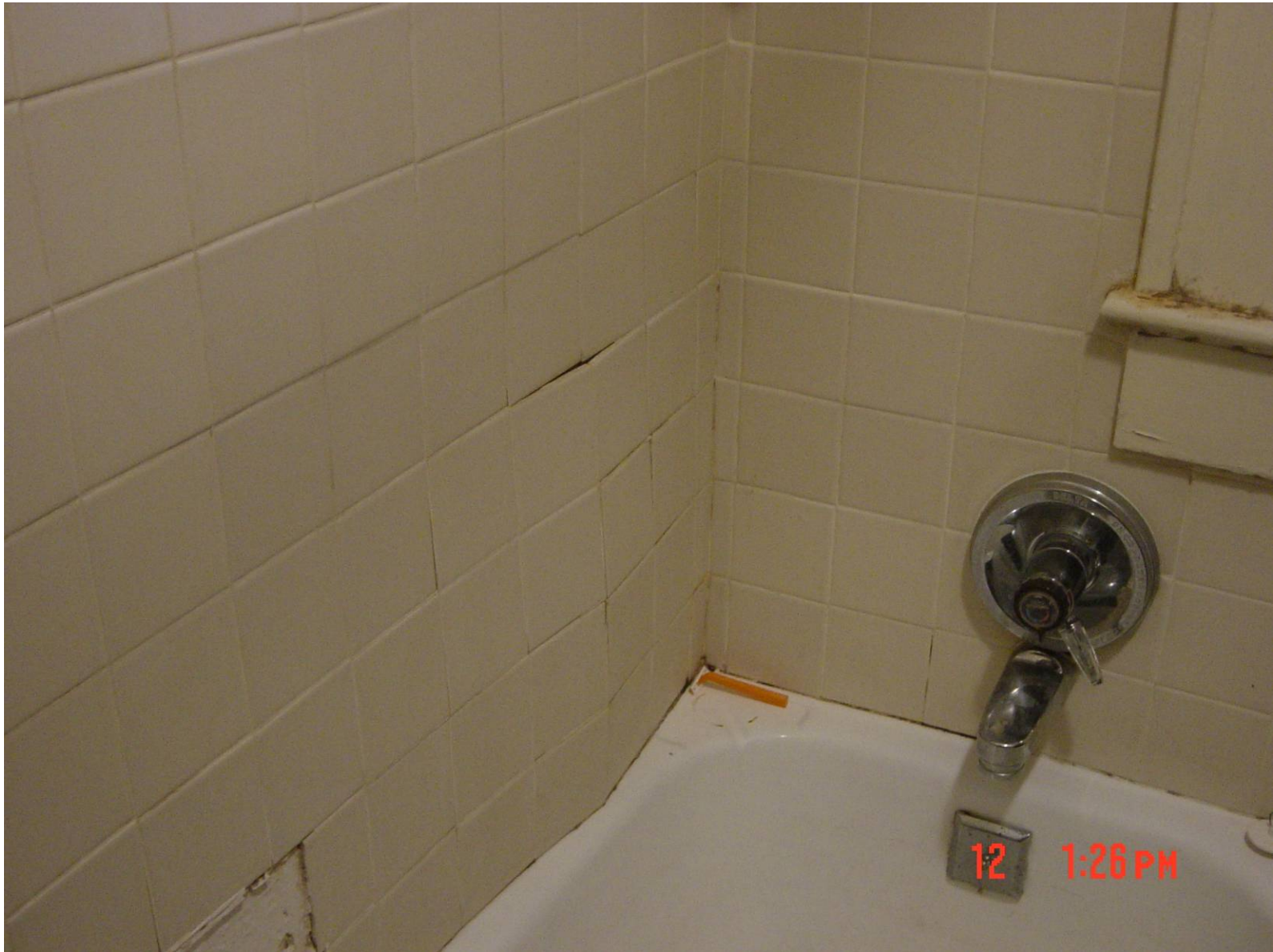
Exercise 5: Identify the Moisture Problems
