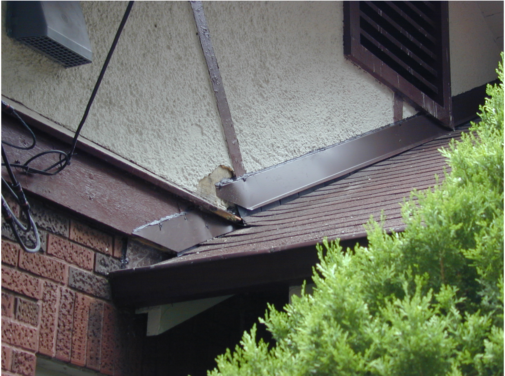
Exercise 5: Identify the Moisture Problems
