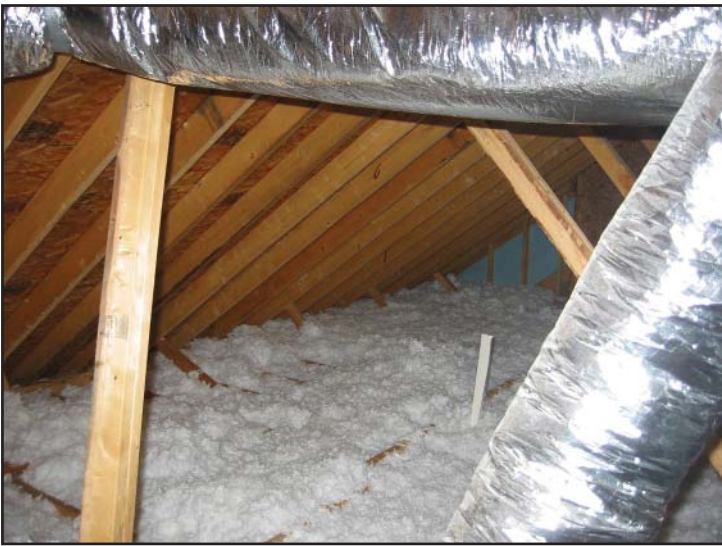
Figure 7.2. Blown Attic Insulation
