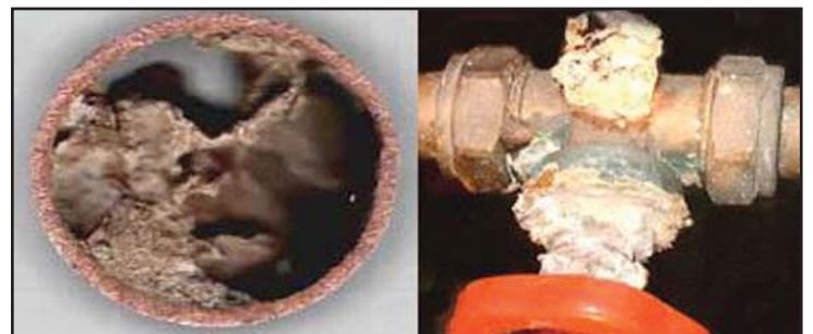
Figure 7.6. Corrosion in Piping Resulting From Galvanic Response
